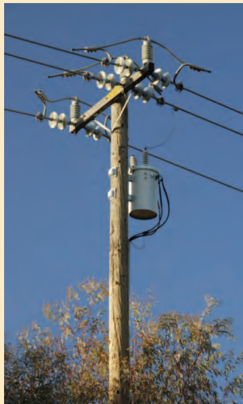
Figure 10.27 A residential utility transformer. (tomba/iStockphoto)
